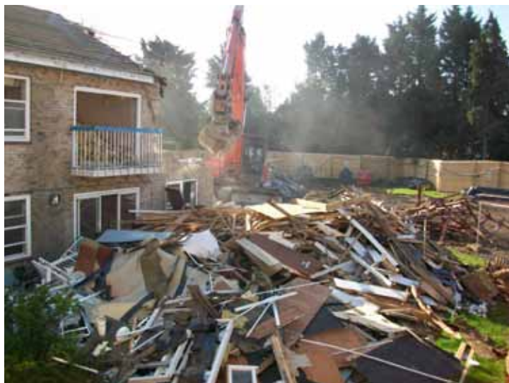
Demolition of the current nursing wing that will be used as the site for the East Wing.
